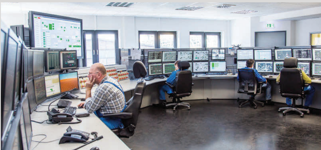
Figure 29: Control room of a Carbon Black plant
