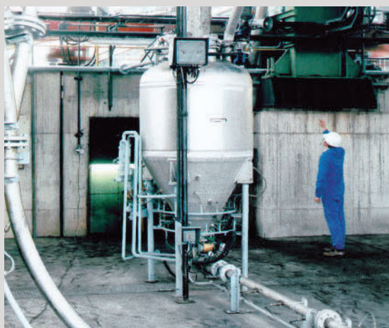
1) Pneumatic conveyor system for Carbon Blacks
